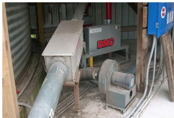
KLEENair spliced into an auger
