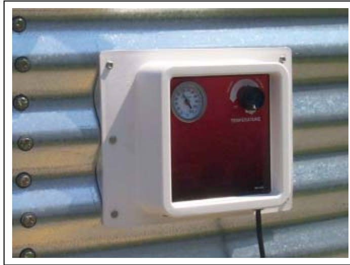
Figure 4G Plenum thermostat mounted on bin wall.
